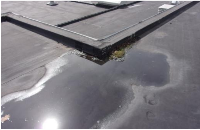
Photo 5 Wylie Elementary School February 2023 Area A: Ponding/vegetation
